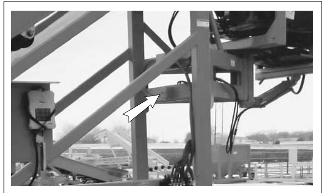
Fig. 7 EMERGENCY STOP - OPERATOR'S STATION
