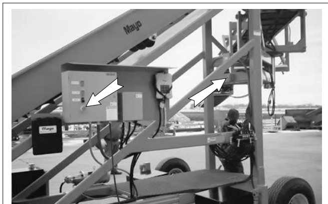
Master Control Panel / Frame
