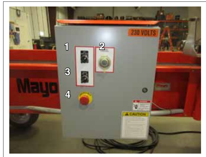
FIG. 4 SCALE CONVEYOR CONTROLS
