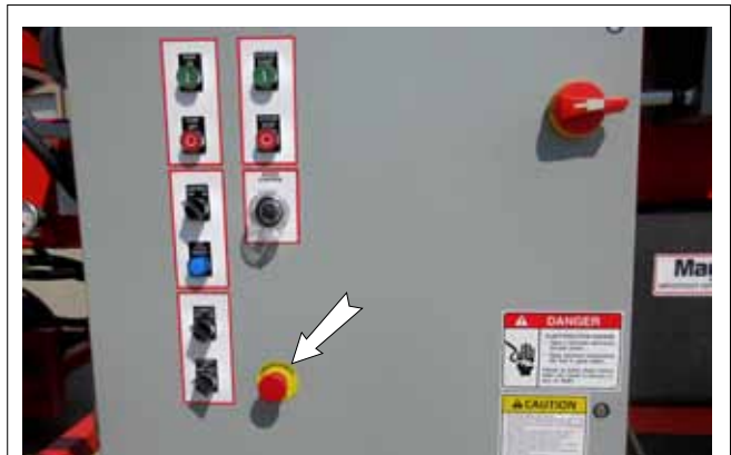
Master Control Box
