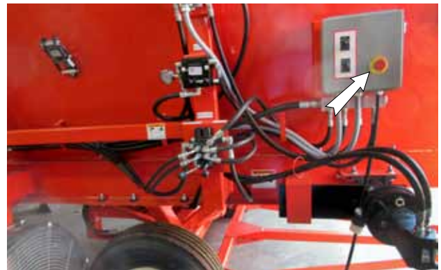
Discharge Control Box
