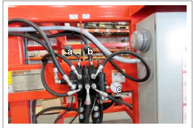
FIG. 7 CENTER VALVES AND GAUGES
